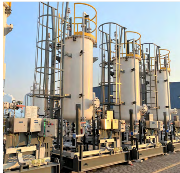
BAB INTEGRATED FACILITIES End User:ADNOC
