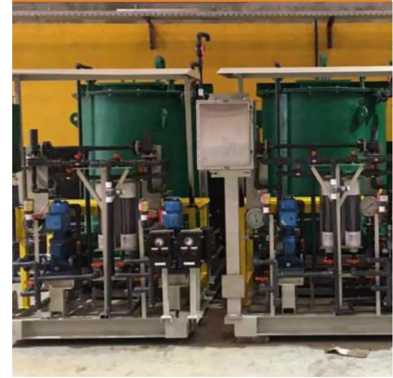
GPIC REFINERY UPGRADATION End User: GULF PETROCHEMICAL INDUSTRIES
