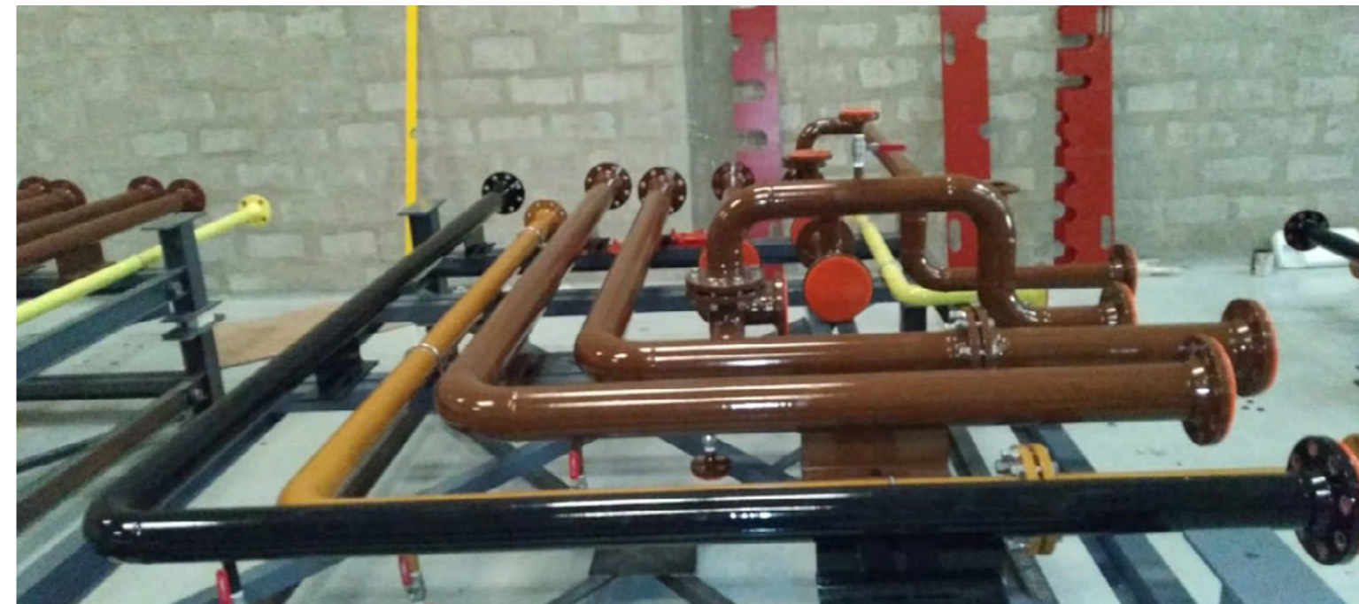
Pipings & Pipe racks
