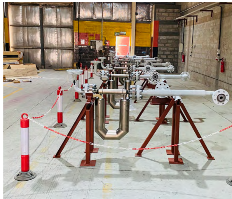
Flow Metering Skids
