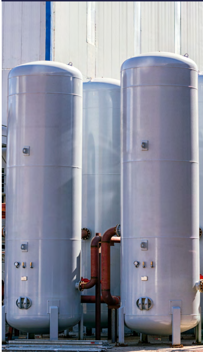
Storage tanks & Vessels
